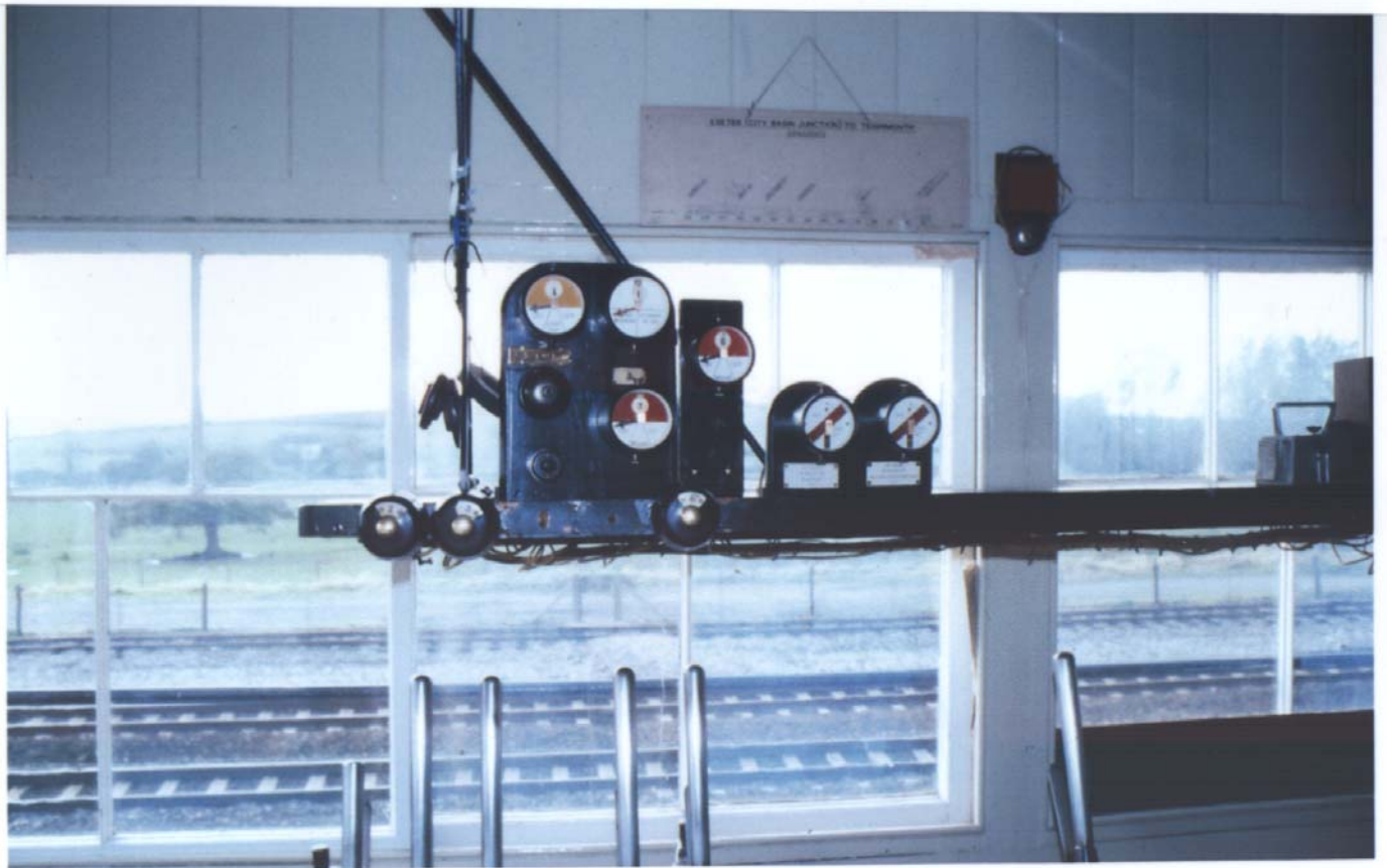
Repeaters on the block shelf at the Plymouth end of the frame.
